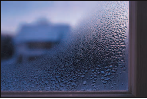
Condensation on the inside of a window-pane.
