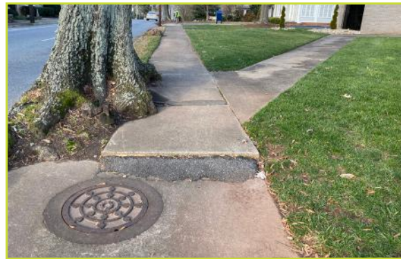
While sidewalks are present along many streets, some are impeded or require repairs.
