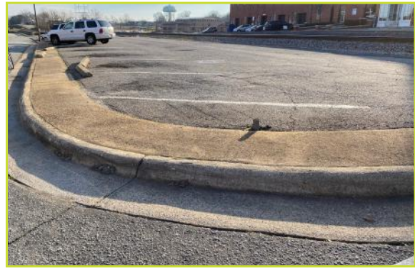
Sidewalk lacks curb ramps and does not meet ADA-accessibility standards.
