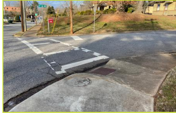
The sidewalk transition to curb ramp is sometimes narrow and does not meet accessibility standards.
