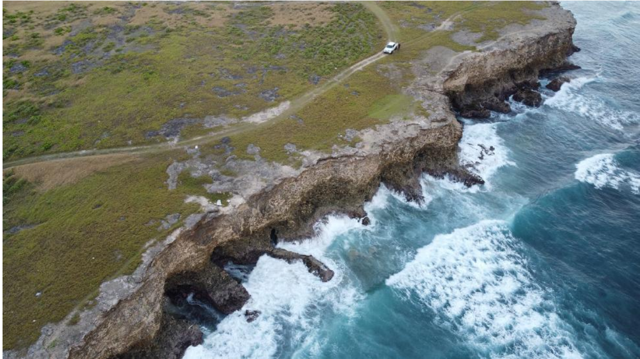
Photo 4. This photo shows the cliff edge and cliff edge undercut.
