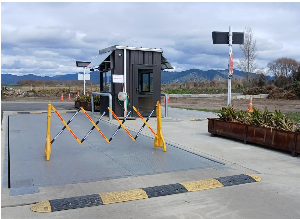
Ōpōtiki Resource Recovery Centre weighbridge ready for annual calibration
