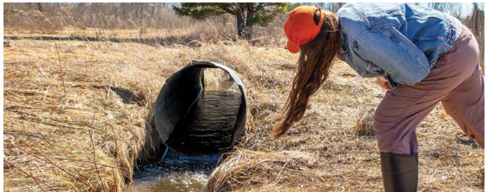
One of eight undersized or abandoned stream crossings gets a closer look.
