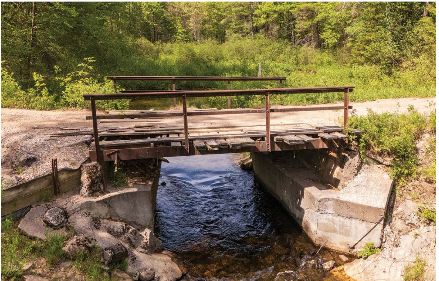
Before: A dilapidated bridge slated for replacement at Fife Lake Creek and Ramsay Road.
