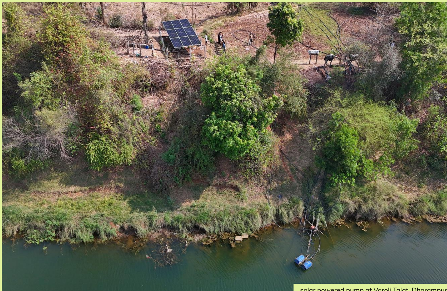
solar powered pump at Varoli Talat, Dharampur
