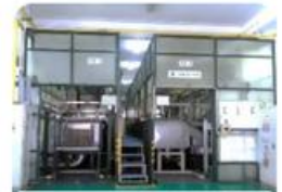
Metal Stripping Line
