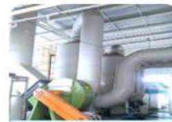
Waste Air Treatment
