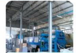
Waste Water Treatment
