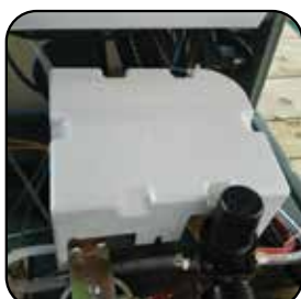
Power protection cover for safety
