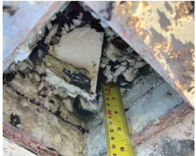
Over 50mm (two inches) of standing water inside a TPO roof assembly. Photo credit: RJC Engineers.
