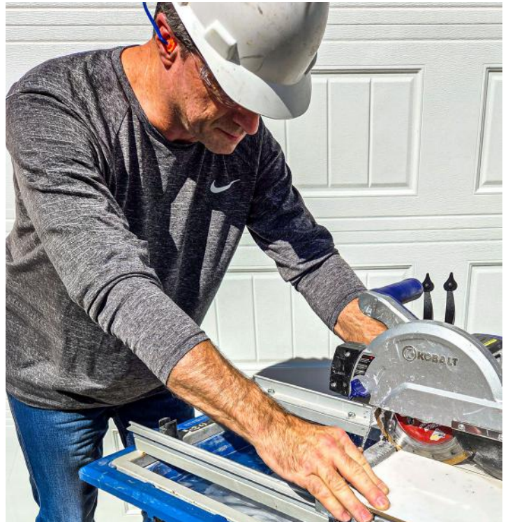
Executing Table 1 compliance: The operator is equipped with proper PPE (safety glasses and hearing protection) while utilizing the primary engineering control.
