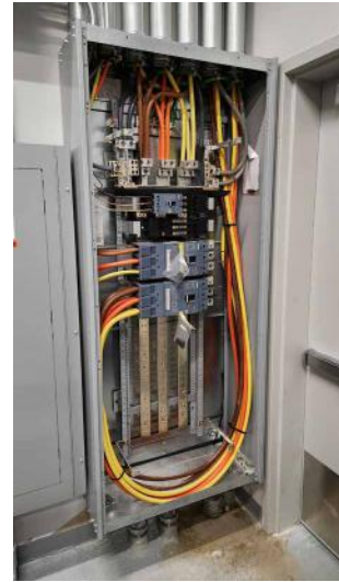
FIGURE 3-21 PV system Tie-In Panel
