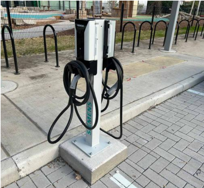
FIGURE 1-51 EV Parking Charger
