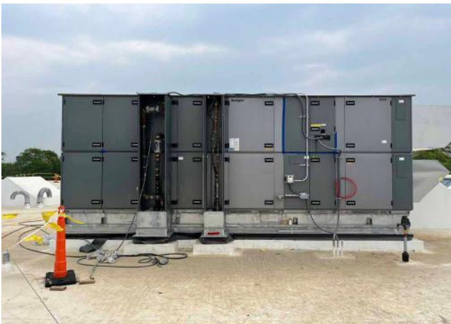
FIGURE 5-07 Swegon DOAS units
