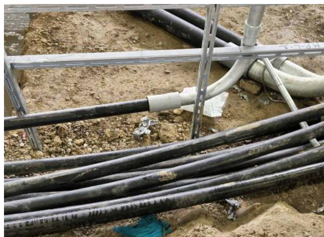
FIGURE 5-05 Non PVC below grade conduit.
