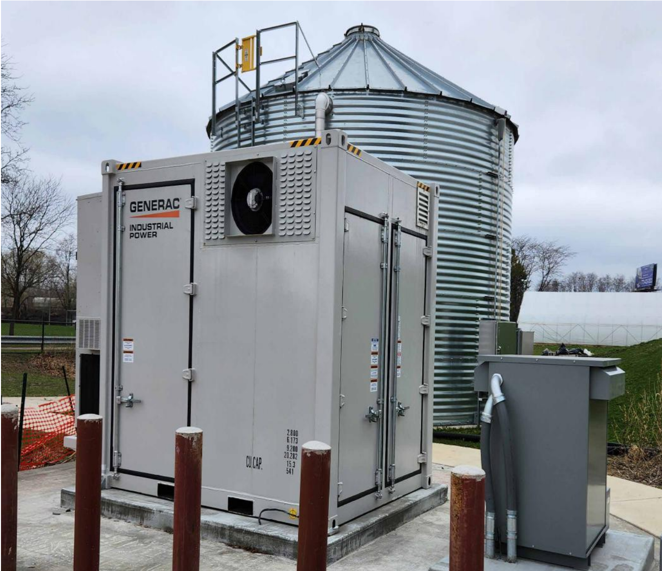
FIGURE 3-04 Battery Energy Storage System
