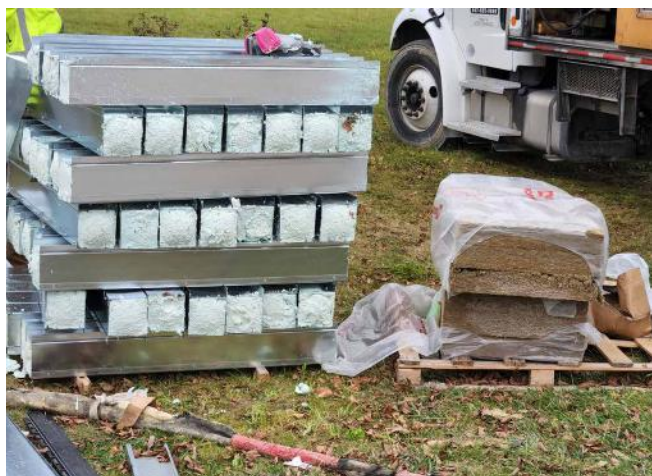
FIGURE 5-04 Insulated CFMF headers on site.
