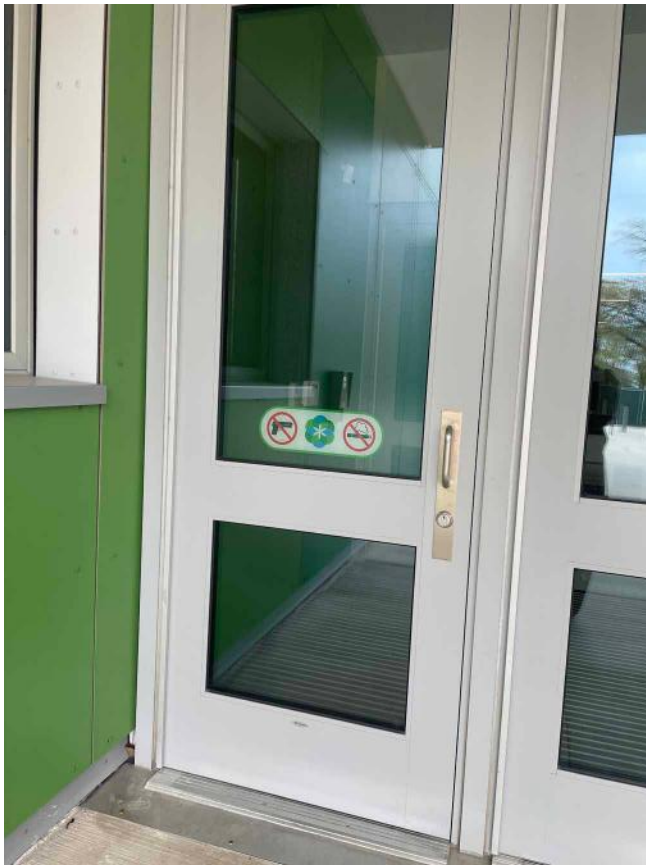
FIGURE 4-04 No Smoking signs at East door
