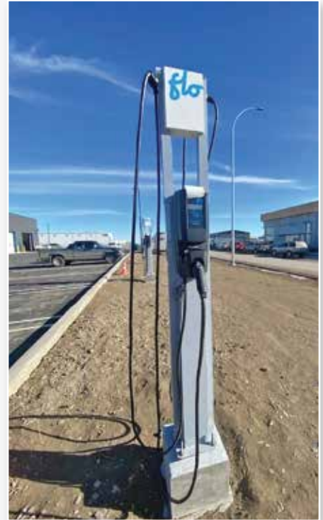
Electric Vehicle Charging. Neu-Lite Electric Inc.
