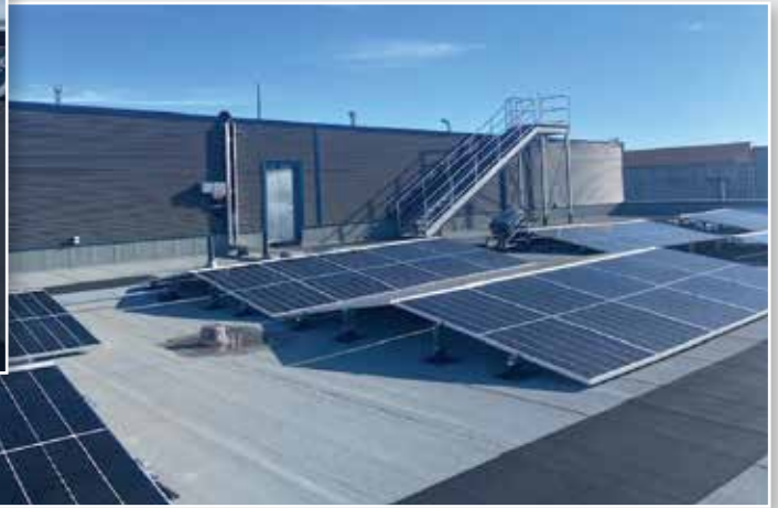
Solar Rooftop. Neu-Lite Electric Inc.
