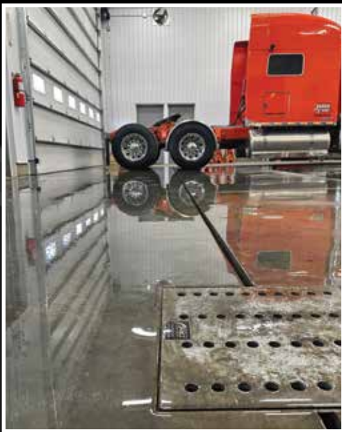
Trench drain in Janam Farms in Diamond City, AB.
