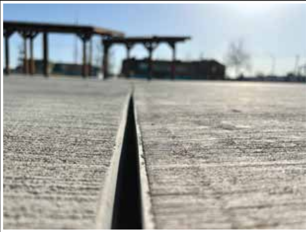
Slot drain in Amundsen Park in Claresholm. Photo courtesy of CT Distributors Inc.
