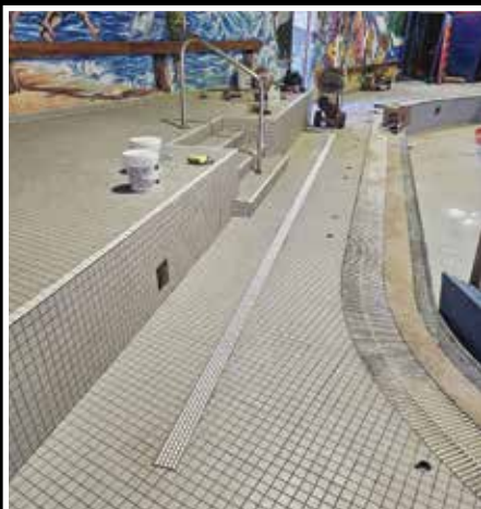
Pool trench drain in Sparwood Aquatic Centre in Sparwood, BC.
