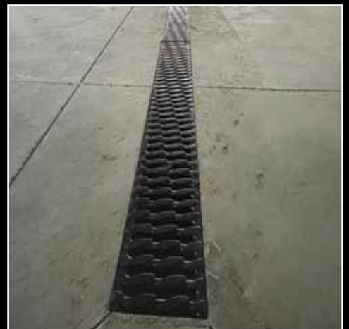
Trench drain in Superform Warehouse, Pincher Creek, AB.
