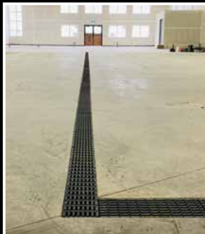
Trench drain in Sunbelt Rentals, Lethbridge.
