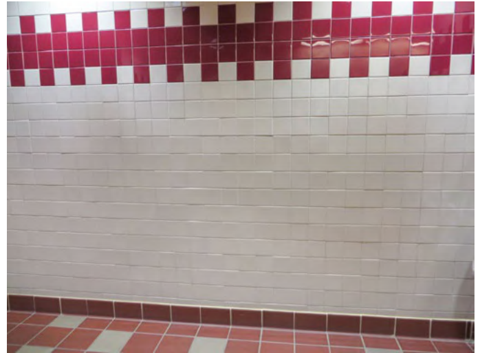
Critical lighting exacerbates the unevenness of the wall that did not meet the ANSI requirements for flatness. With the lights turned off, the tile looks great.
