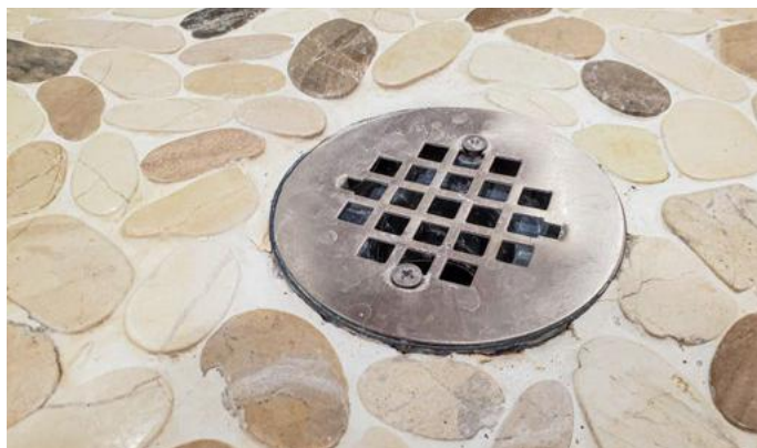
Some of these pebbles are flat while others are slightly rounded, but notice that the grout joints are significantly lower than the edge of the pebbles.
