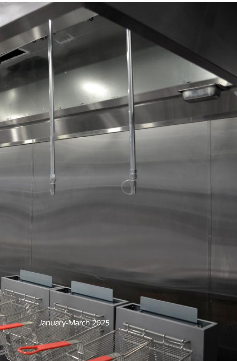
Fire suppression system components like nozzles need to be cleaned routinely to prevent buildup of flammable product.
