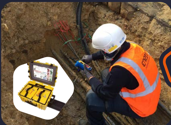
De-energized and dual grounded.
