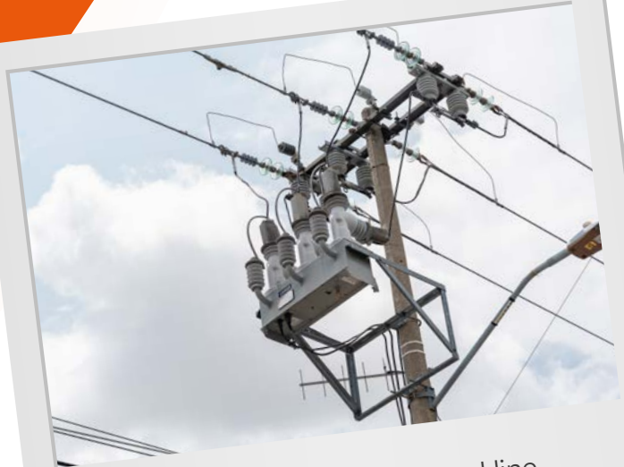
Medium voltage overhead line
