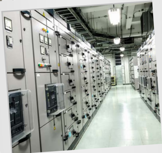
Medium voltage substation
