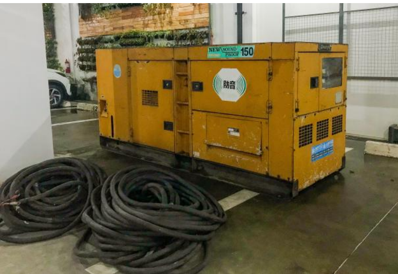
A diesel generator typically used in the Philippines
