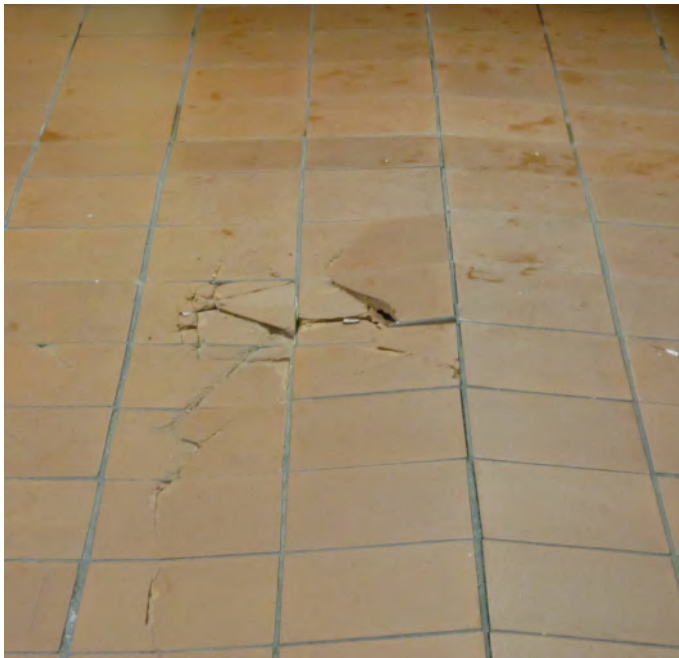
Without the design professional's details on the location of the movement joints, the tile installation can fail. As seen in this image, no movement joints were specified and the 6" x 6" quarry tile failed, resulting in tented tile.
