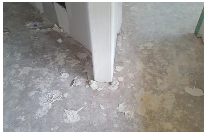
Unfortunately, as seen in this image, many jobsites are not clean and free of contaminants as described in this standard. These materials must be appropriately removed before installing tile.
