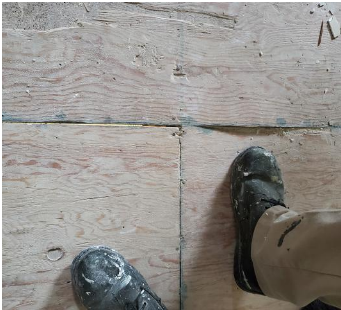
This is an example of a non-compliant subfloor. The 1/2" three-ply plywood does not have a tongue and groove running along the long dimension, nor any wood blocking to support the sagging joint.
