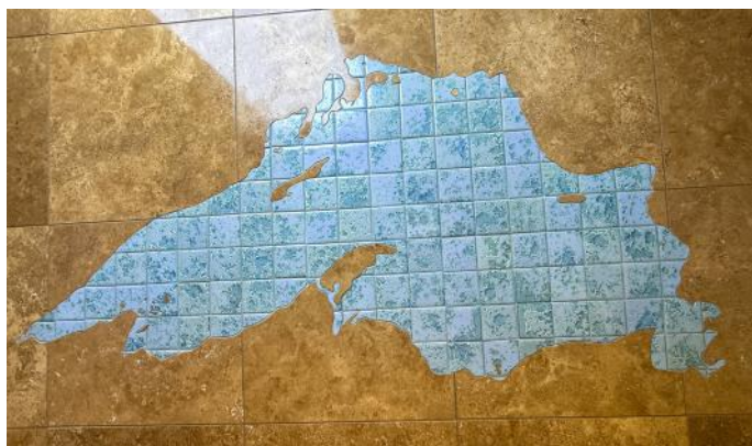
Mosaic cleaned and grouted. Note crooked joints and alignment
