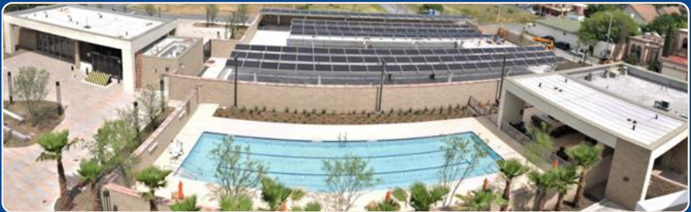
Photo Voltaic Panels installed on staff parking canopies.
