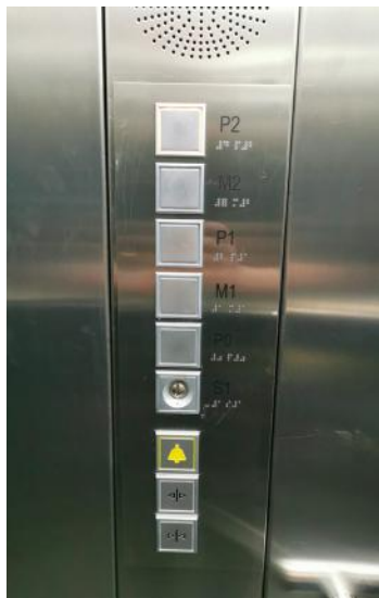
Ascensor D / Lift D
