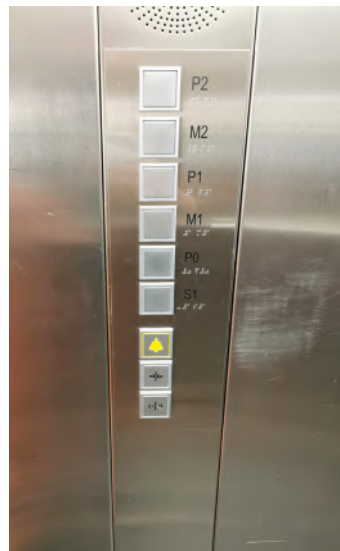
Ascensor B / Lift B
