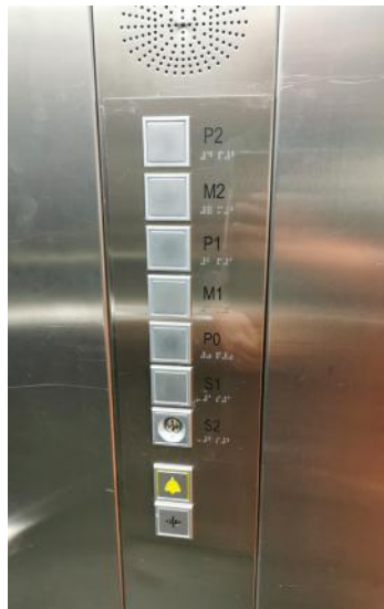
Ascensor C / Lift C
