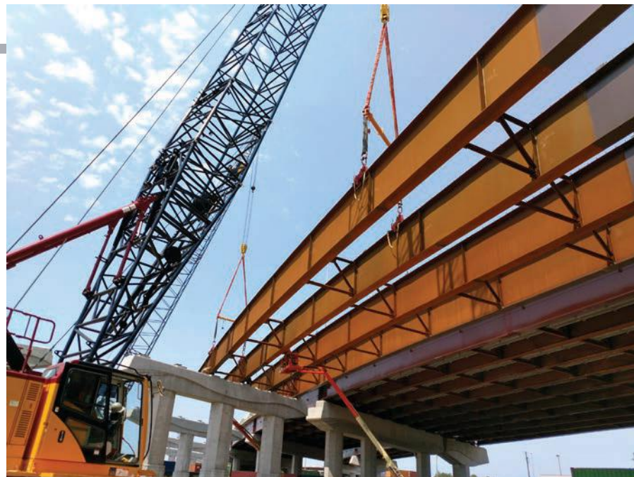
The stability of a spreader beam is a result of taller headroom.
