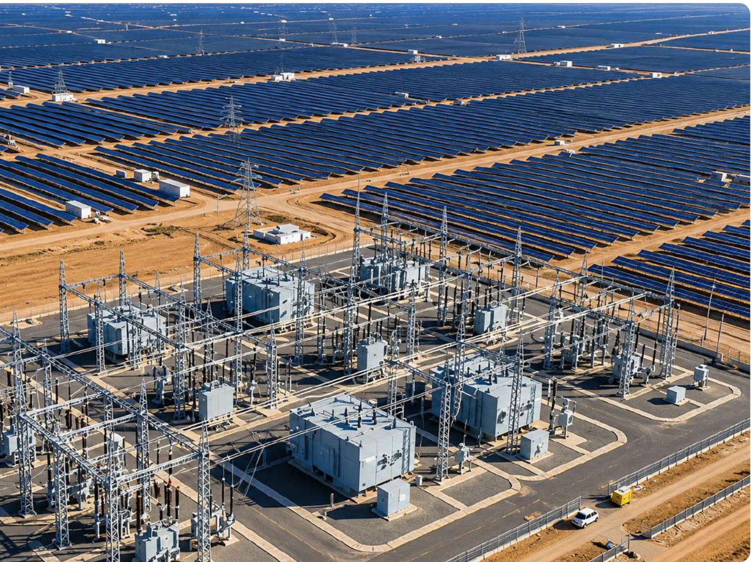
A high-voltage substation amid the vast solar fields of Khavda, Gujarat, supporting one of the world's largest renewable-energy projects. The 30 GW project is targeted for completion by 2029.
