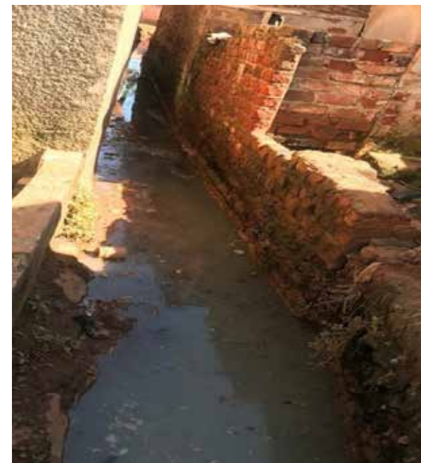
Image 7.4: poor drainage and flooding
