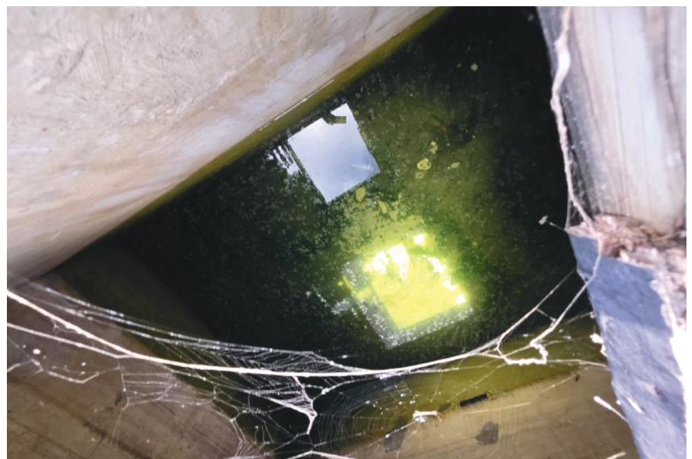
An out of commission tank, one of which has been earmarked to receive water from the RO Plant
