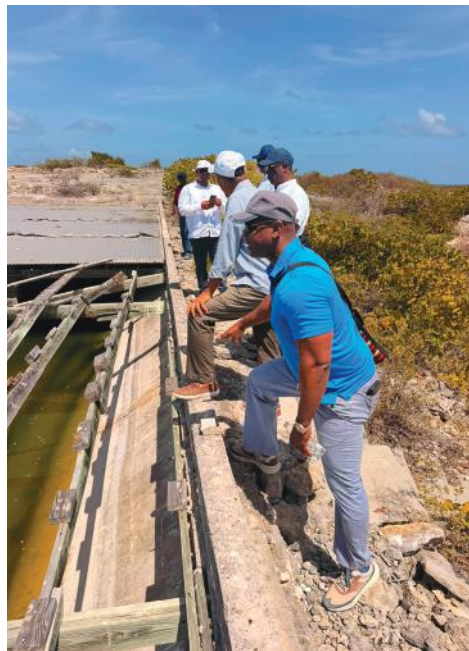
PDM Executive Members examine a seemingly disrepair catchment tank on Salt Cay
