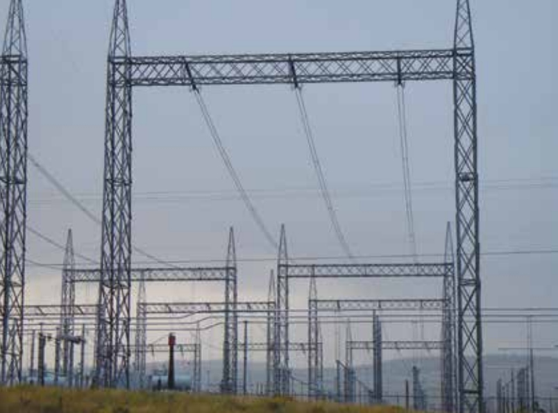
BC Hydro Nicola Substation.
