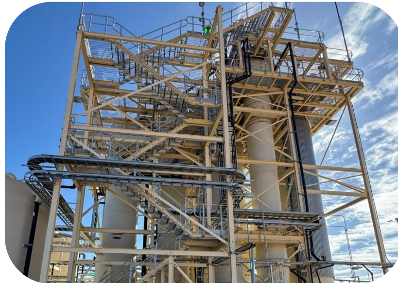
Heathgate's new ion exchange elution plant (U-column)
