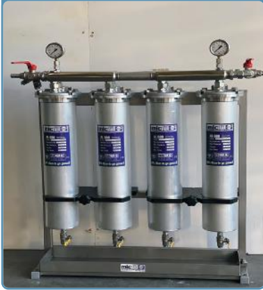
FUEL FILTER SYSTEM
