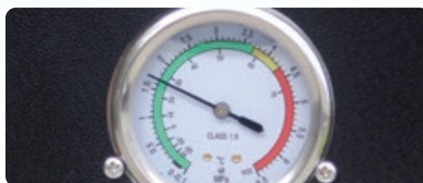
Refrigerant System Pressure Gauge
