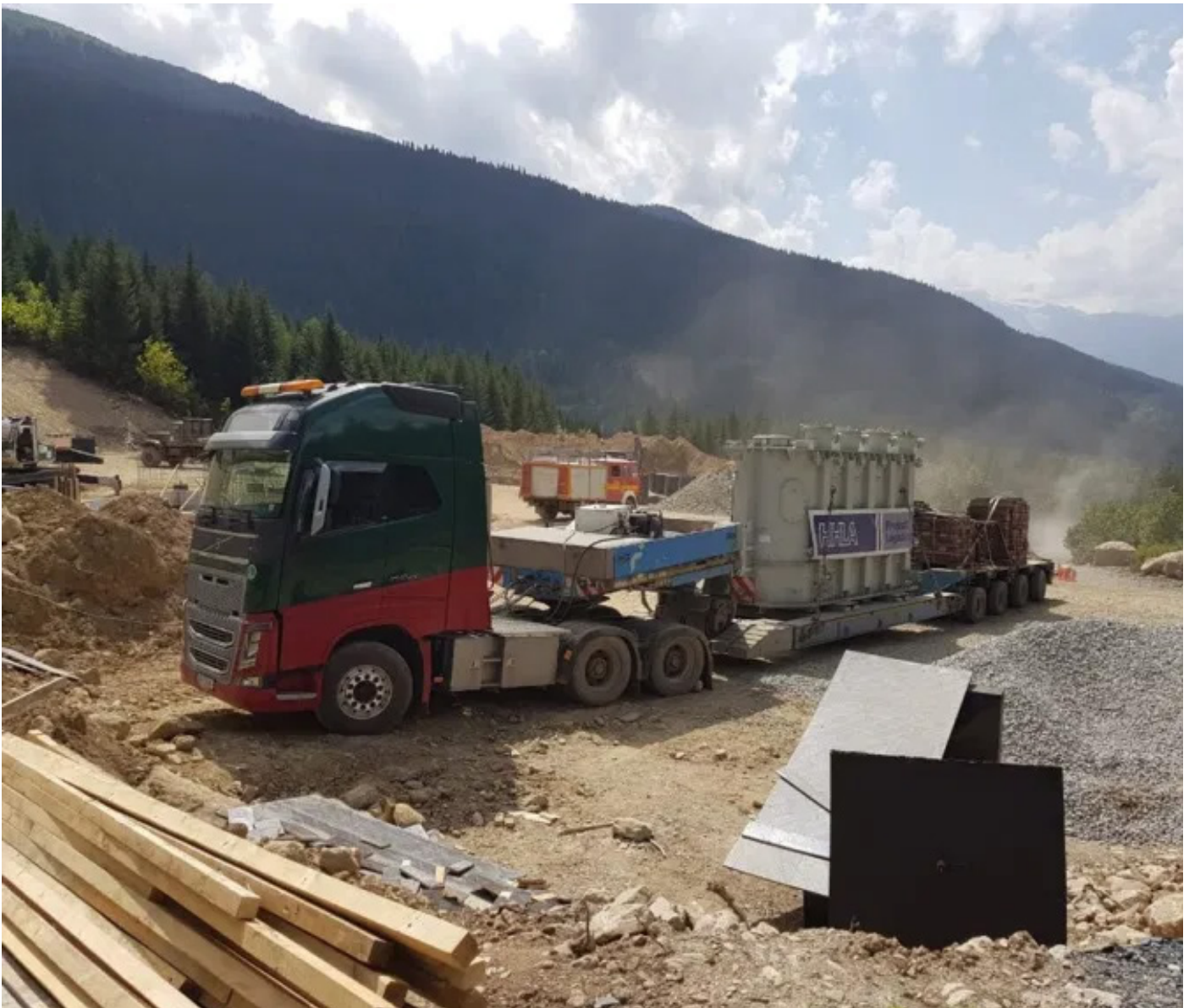
HHLA Handling a Transformer © HHLA / Thies Rätzke
