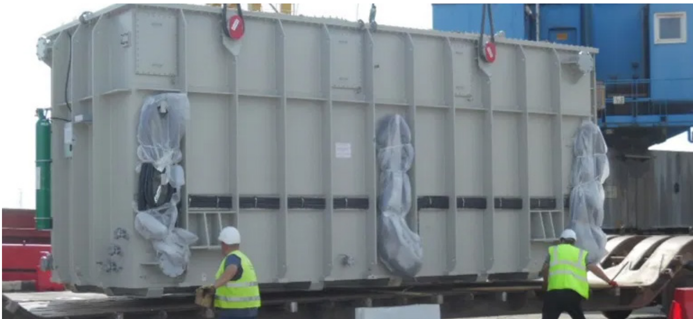
Transformer Under Hook © HHLA / Thies Rätzke
