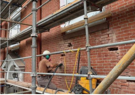
Worn brick comes out of the Washington Street wall, course by course.
