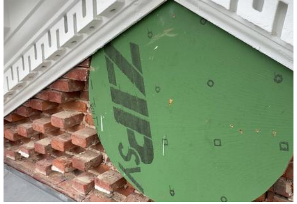
The pediment, opened up where the brick had failed.
