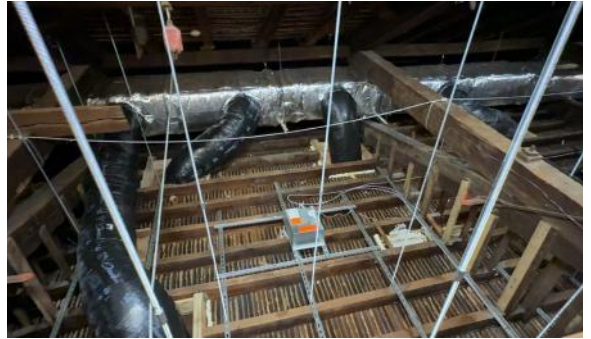
New ductwork is installed and insulated.
