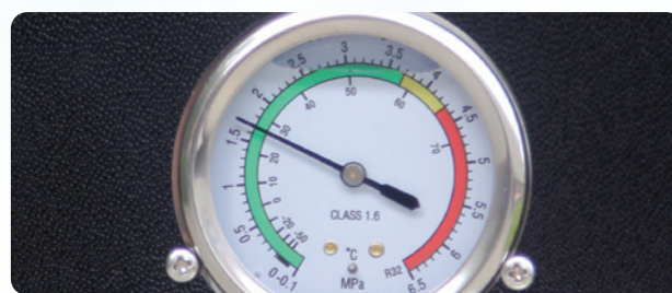
Refrigerant System Pressure Gauge
