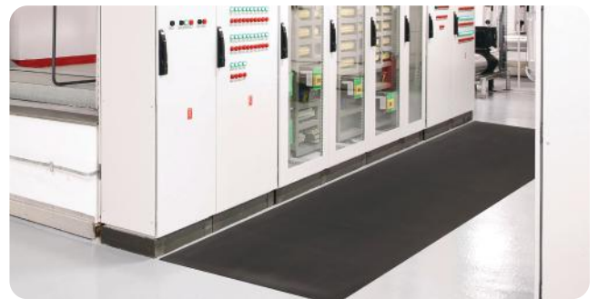
Electrical Safety Matting
