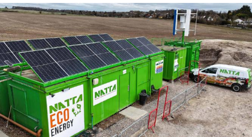
Solar PV/Battery Storage System for Natta Welfare Units at our Sittinbourne and Manydown Sites
