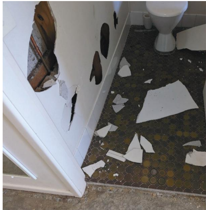
Photo 1. Damage wall lining containing asbestos materials.
