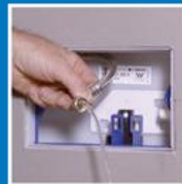
Flush water supply
